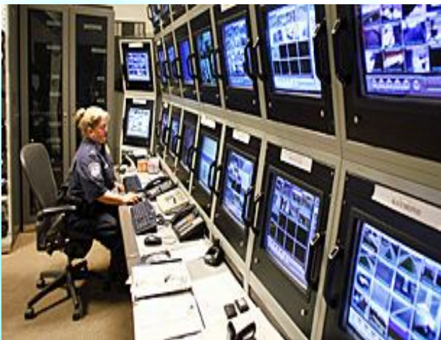
Public safety command communication
